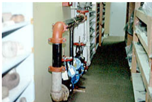
High risk storage location (next to water valve). Photo courtesy of the Art Conservation Center @ Univ. of Denver (formerly RMCC), Denver, CO.
